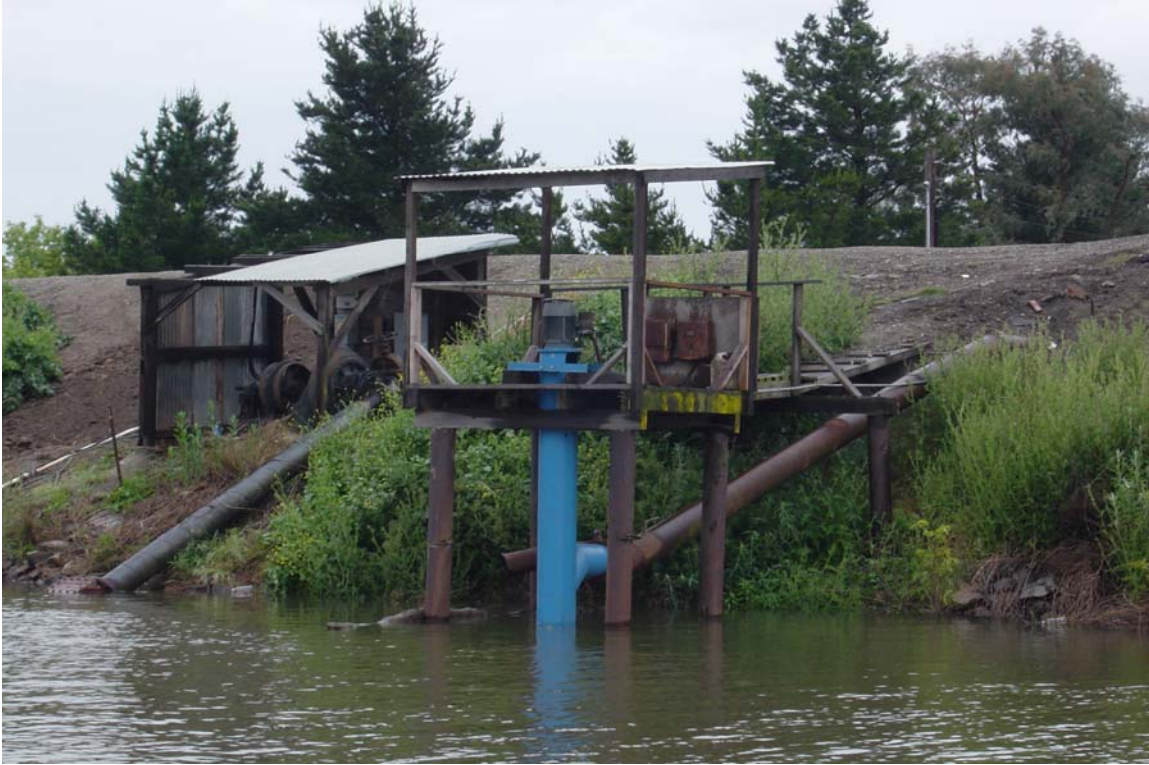
Figure 10: The water diversion pump at the Stockton Brick Company.
